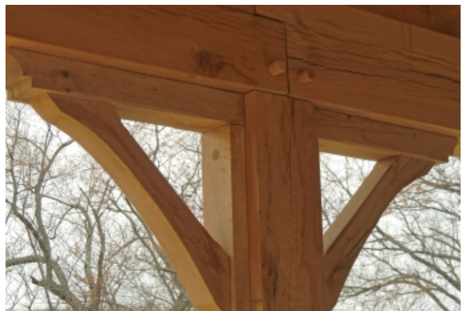
Heavy oak timber beams will age gracefully in place, exactly what the owners wanted
