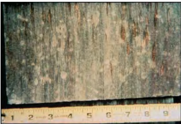
c) Many small hail impact marks, but no splits in shingle
