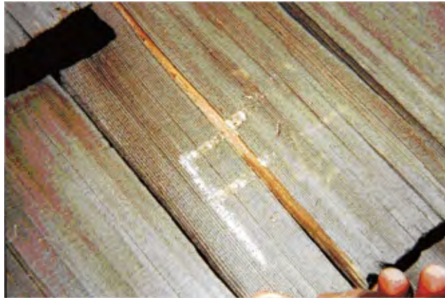
e) Footfall split damage (note no denting and new cedar color)
