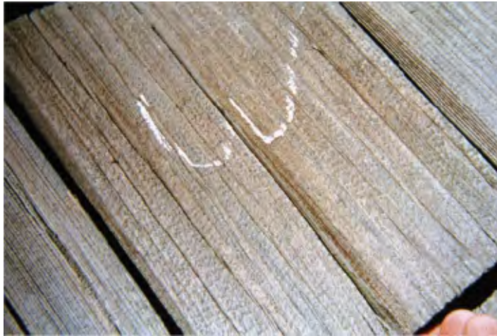
Photo courtesy of Haag Engineering Co.
