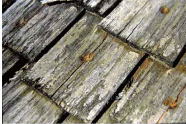
d) Intentional ballpeen hammer damage (note regular pattern)
