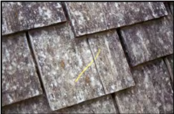
b) Weathering split and small hail impact marks
