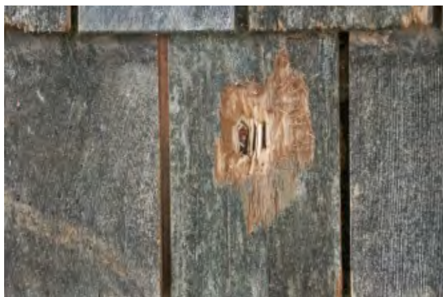
f) Actual pressure washing damage (... yes, it really is!)
